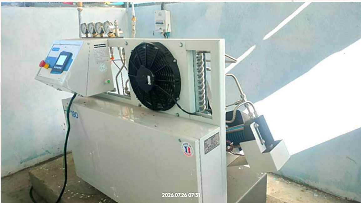
Installation of "Oxygen Booster Pump" at District Hospital Thoubal under the MoHFW Gol. ( Refiling & storage of Oxygen Cylinders )
